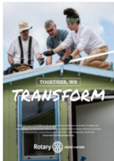
Rotary members work together to build the roof of one of the tiny houses donated by the Rotary Club of Mercer Island.
